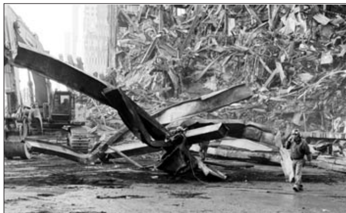
Workers remove twisted steel and other debris from the World Trade Center site. (Photo by Shawn Moore, Occupational Safety & Health Administration, U.S. Department of Labor.)
